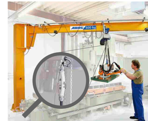
Jib crane with additional power socket and plug on hoist (Fig. 13)
